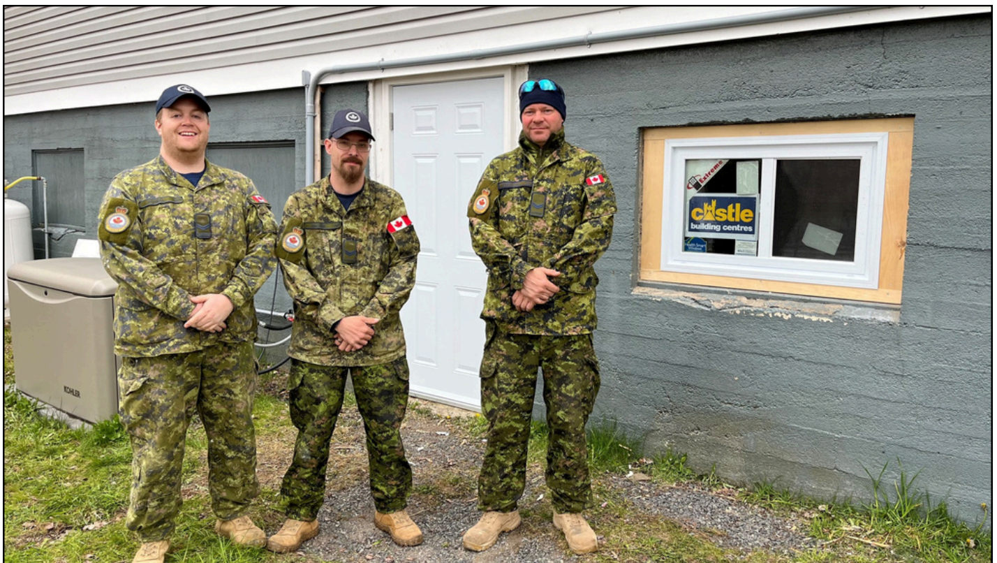
Members of the Construction Engineering Flight 144 in Pictou are putting in some new windows and doors at the Hillside Community Hall this week. From left are: Cpl. Kodie Powell, Cpl. Travis Decker and Cpl. Greg Creighton.
