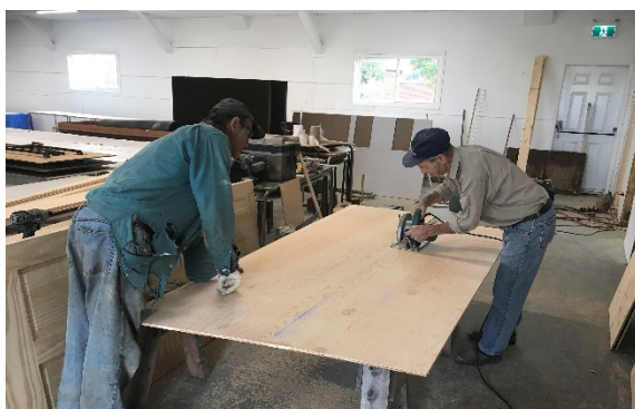
Sandy Townsend and Hugh Murray continue with maintenance work in the Kinsmen Building on the Pictou Exhibition Grounds.
